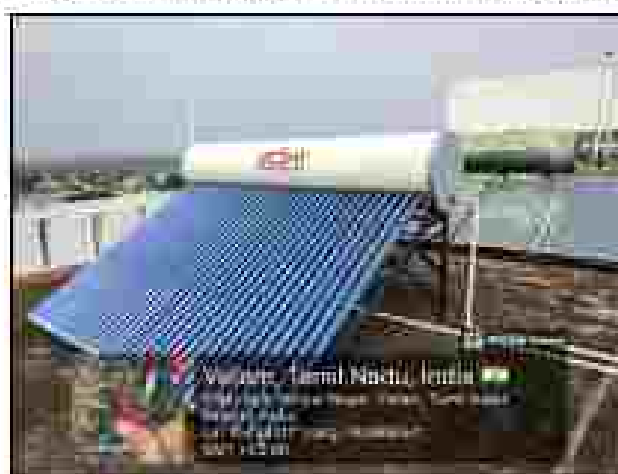
Solar water heater observed in the campus
