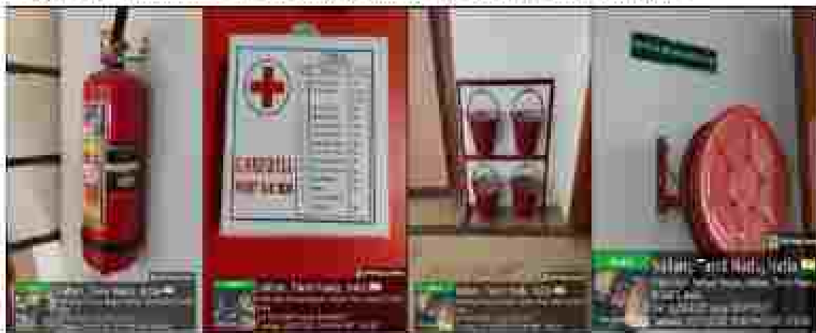
Fire safety measures and first aid kit were observed inside the campus
