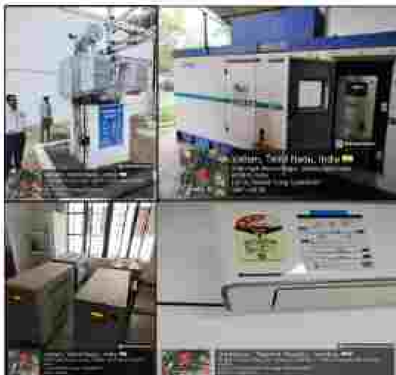
Energy conservation facilities observed in the Campus
